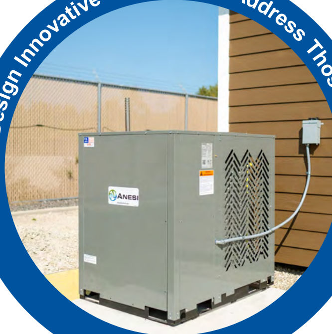
Gas Heat Pump installation at Peoples Energy Training Center
