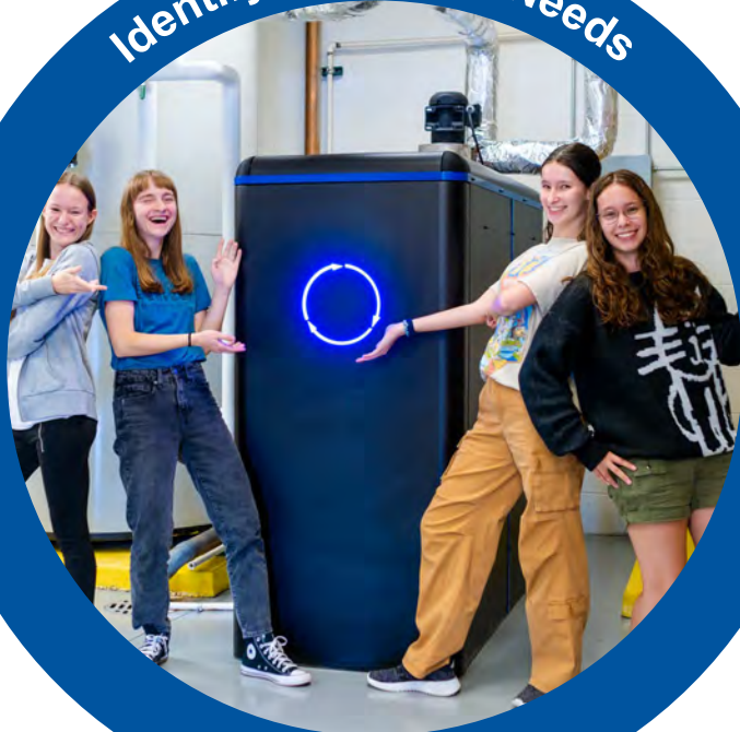
Carbon capture with heat recovery technology installed at Grayslake High School
