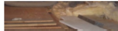
Figure 21331-1: Required attic insulation R-value is a minimum of 49 or the maximum amount with an SIR greater than 1.0
